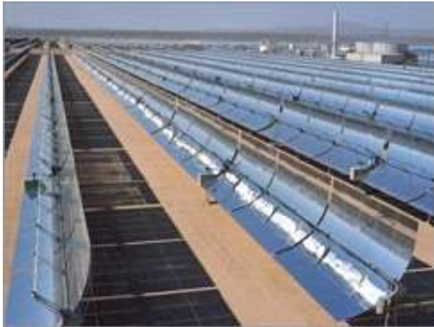
Solarthermisches Kraftwerk Photo: US Department of Energy
